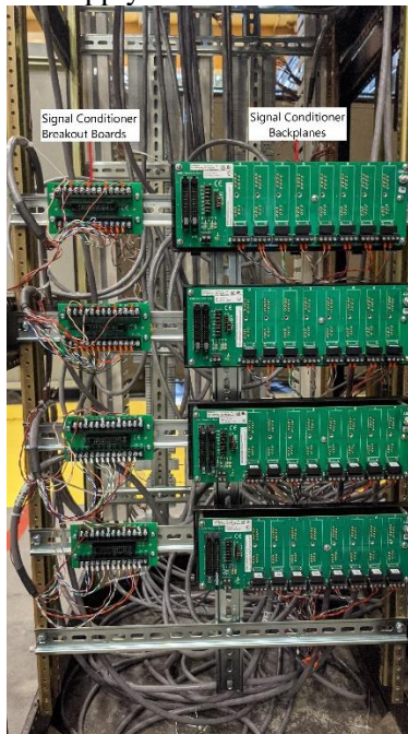
Rack #1 front panel, lower section; signal conditioning breakout boards (left) and backplanes (right)
